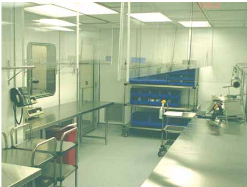
In-dwelling carts may serve as mobile shelving to allow for the smooth transfer of drugs and supplies into and out of the compounding rooms.
